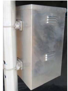
2B enclosure side view showing 4" vents
