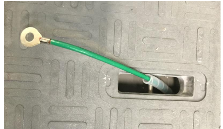
Figure 4 . Top View of Shield Lid with the un-covered Lift Pin Slot and 5' Ground Wire with Spiral Wrap in the in-use position.
